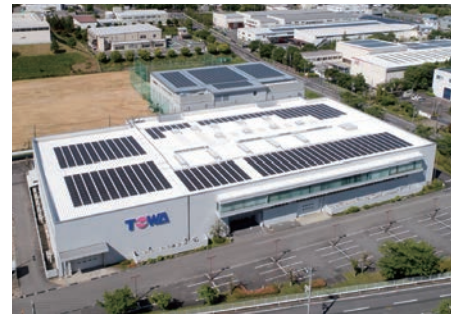
Solar panels installed in an existing building at the Kyoto East Plant (the front building)
